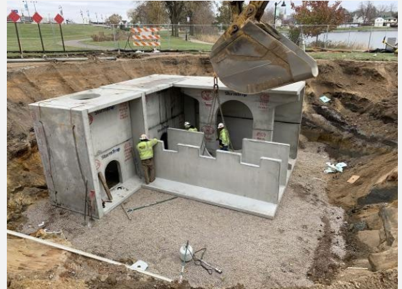
Urban stormwater carries pesticides, oils, road salt, bacteria, litter, leaves, dirt and more down storm drains. St. Cloud's new filtration facility will filter out stormwater contaminants.
